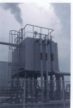
Obama Binary Power Plant
